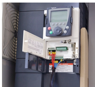
13 / Crane Frequency inverter
