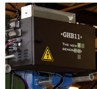
18 / Hoist electric cabinet
