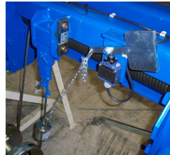
9 / Safety limit block operated
