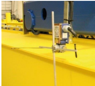
6 / Crane limit Switch
